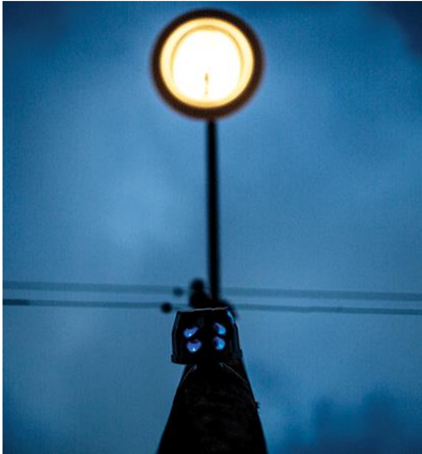
FIG. 3. A lamp post with a motion sensor prepares for lighting to be the smart city's backbone. (Courtesy of Jeppe Carlsen/DOLL)
