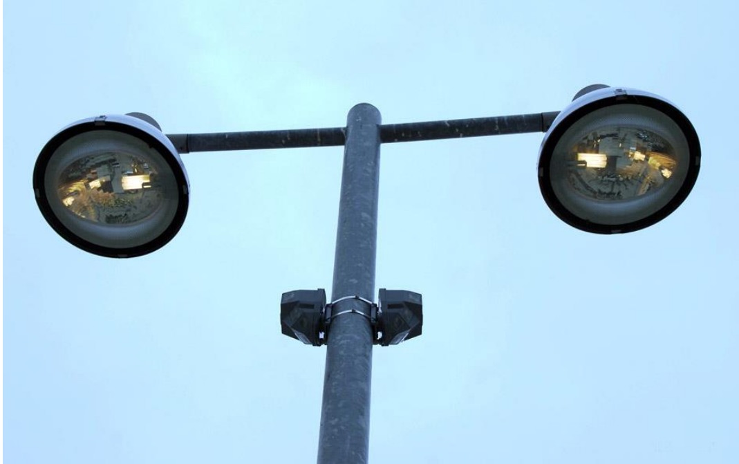
the 'citysense' module powering the concept can be attached to new LED or existing old streetlamps, as shown here
