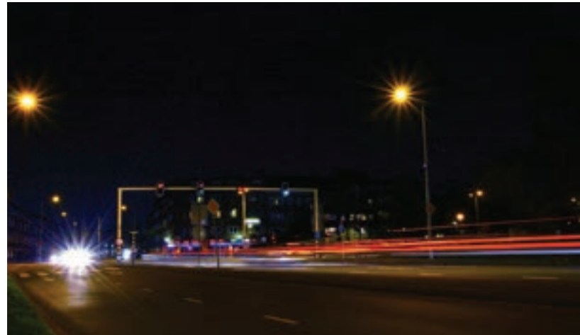
Intelligent streetlights on Vlaardingerdijk in Schiedam
