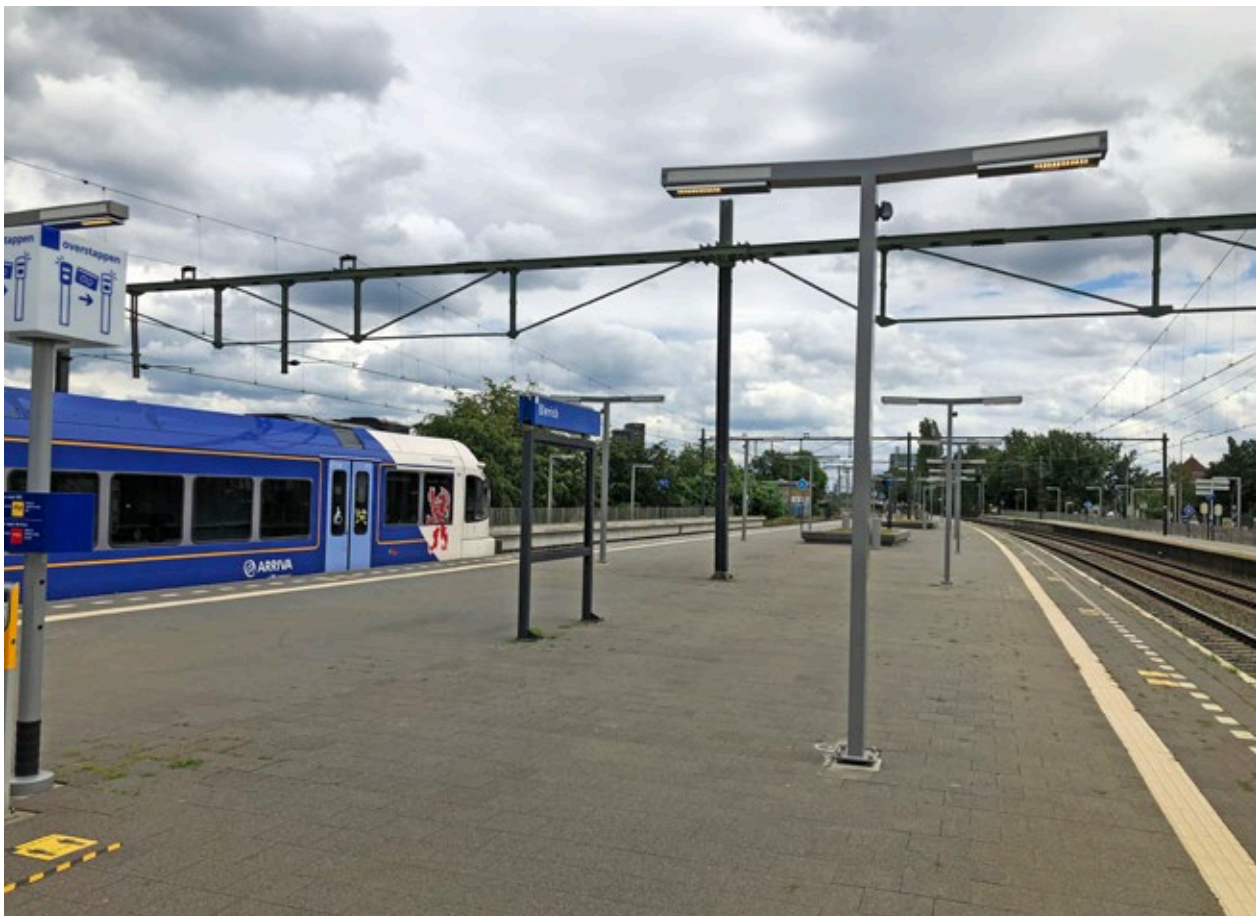
By the final delivery in June 2020, the grey dimming sensors had been installed. Above, 2 speakers per post with double outrigger. Based on what we know today, we would apply one speaker per lamppost on the rail side.
