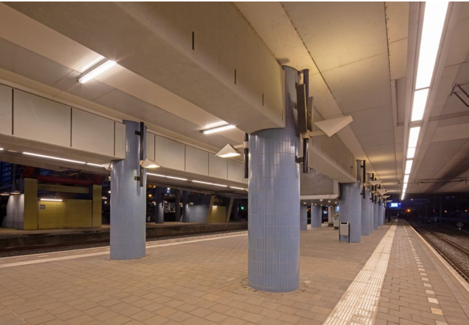
LED lighting at Amsterdam Sloterdijk station
