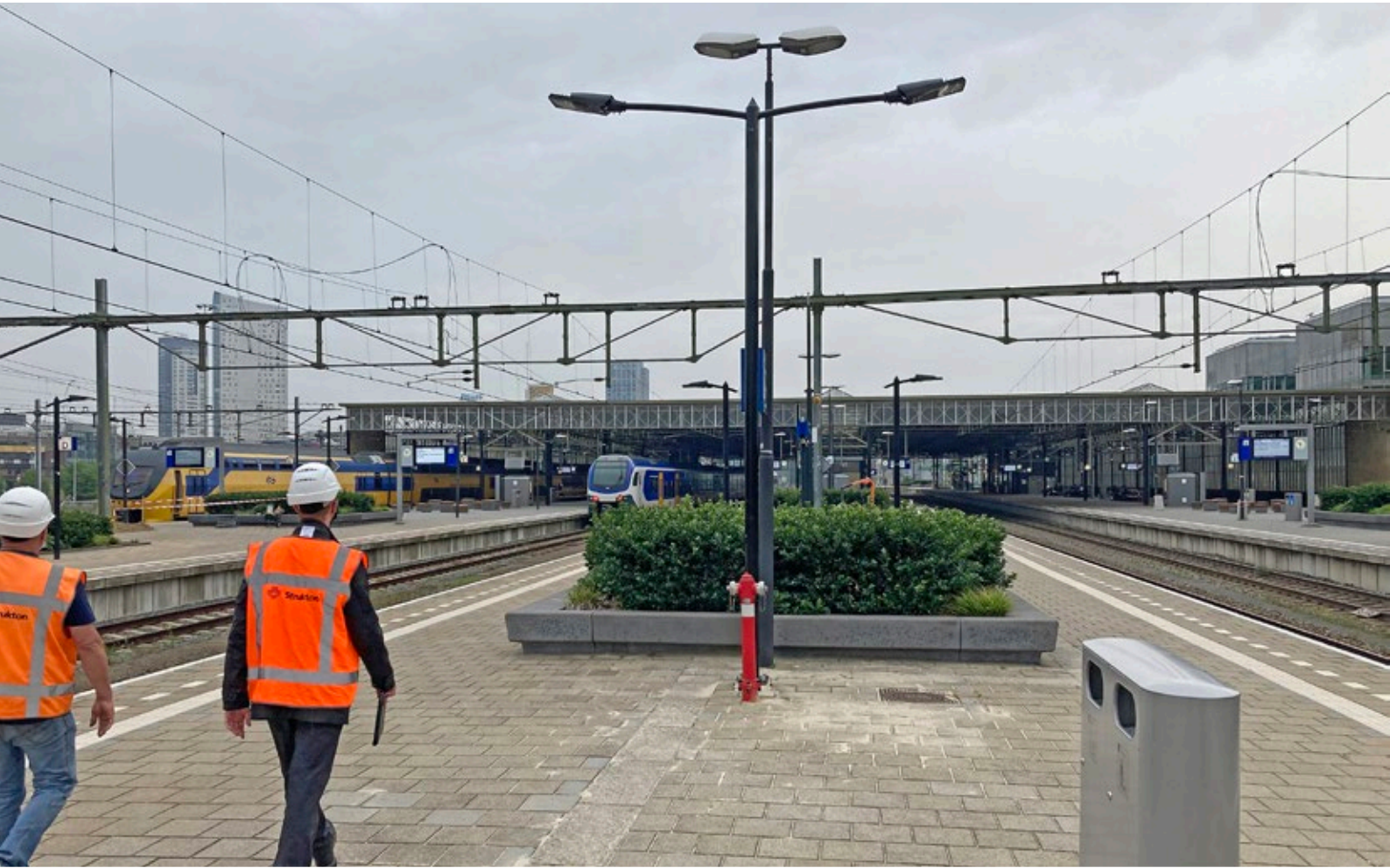
The new post was placed while the old remained to be uprooted.
