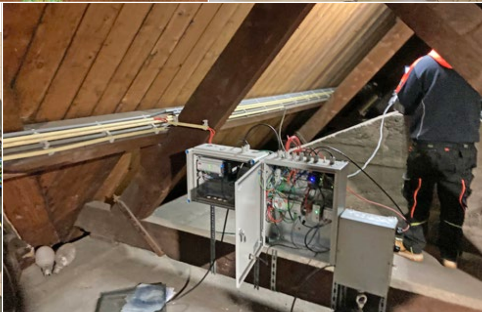
Light controls in the attic above the train hall.
