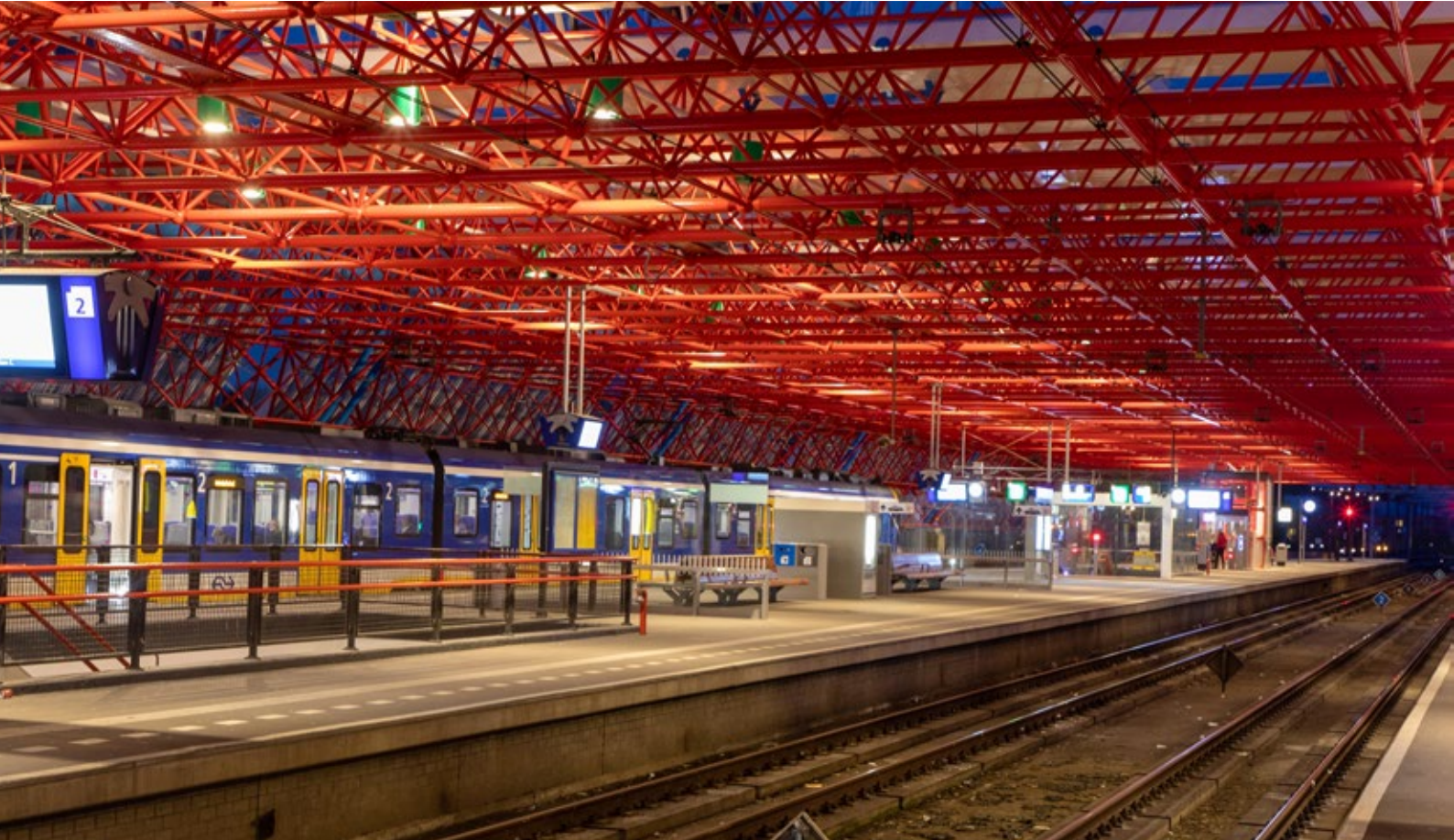
Above: the spotty light on a platform at Almere Centrum station in 2016. Below: The new situation with much higher illuminance and improved uniformity.
