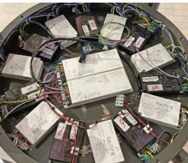
16 drivers in the chandelier. The 2 x 100W TW drivers in the centre were now installed outside the fixture in the attic.
