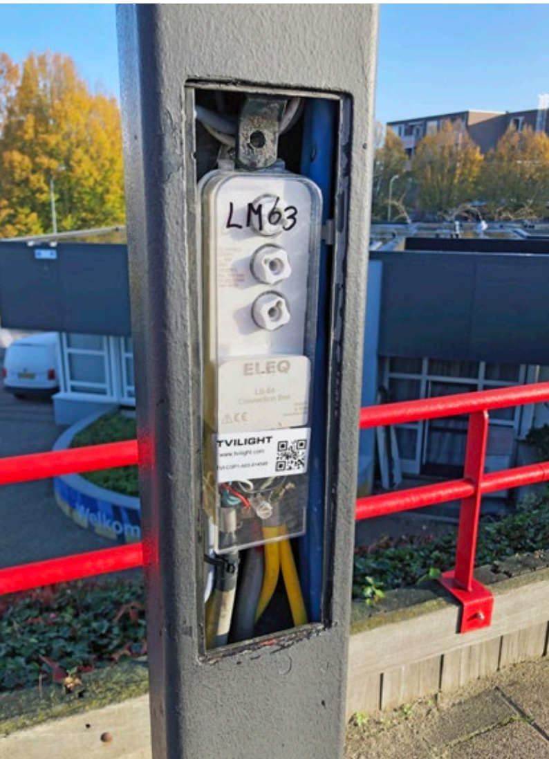
Eleg touch-safe splash-proof junction box in lamppost at Helmond station.
