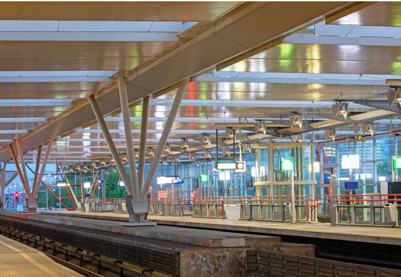
The spotlights between the triangles were converted to a new LED interior.
