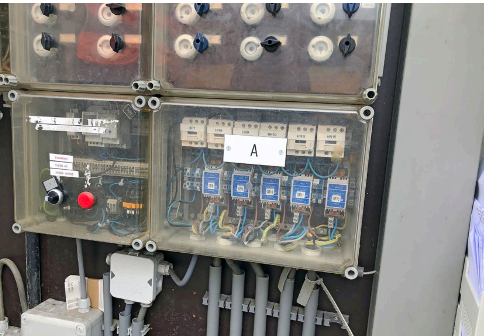
Following the experience in Olst, the switchboard in Blerick was fitted with 5 inrush peak limiters as well. The old fuses at the top. The black and red button on the left are for manual override (for daytime testing of the light).
