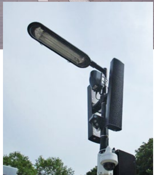
'Totem pole' in Zuidhorn: an old lamppost with a lighting fixture, 2 speakers, a camera and an antenna.
