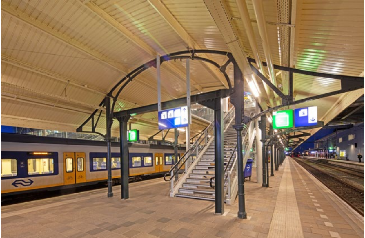
The monumental canopy with the new LED lighting under the new cable duct.
