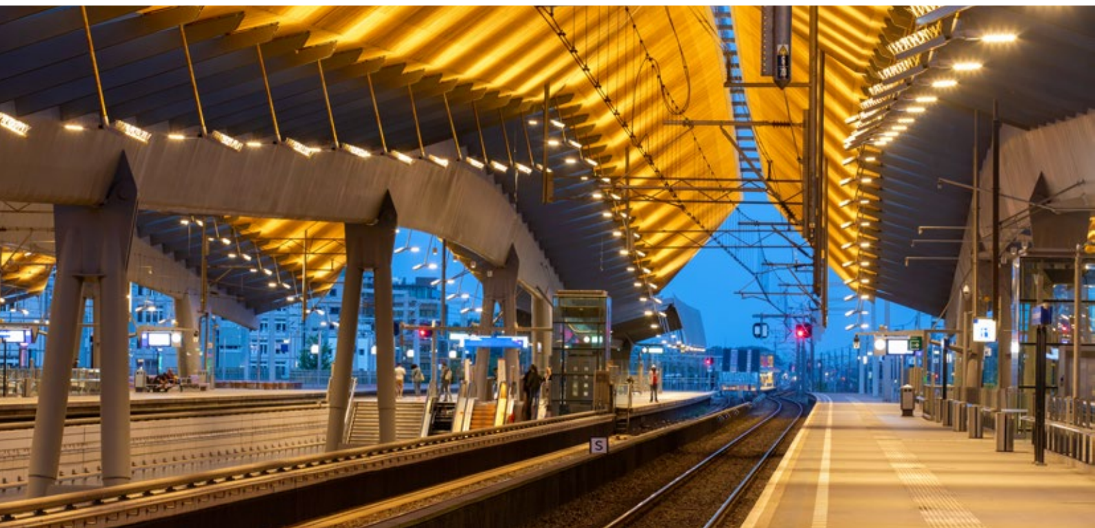
The undulating canopy with its up and downlighters is once again clearly visible after the LED replacement.
