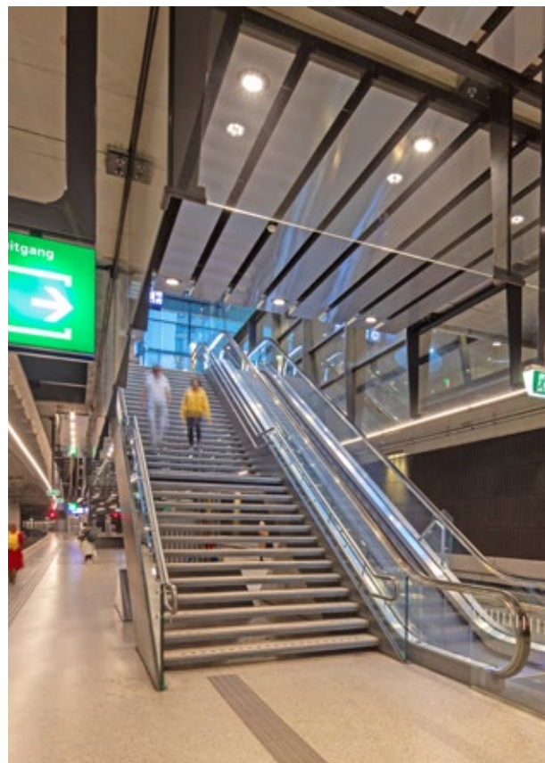
There was too little light on the halfway platform of the stairs. Additional spotlights were installed (behind the slats).
