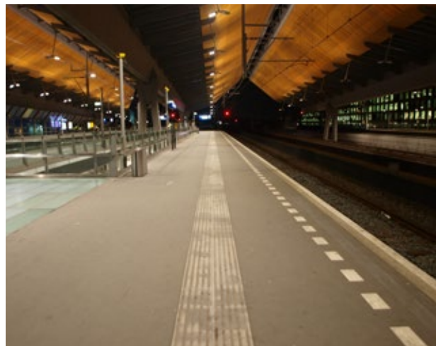
The situation before the LED replacement. A large proportion of the uplighters was faulty.
