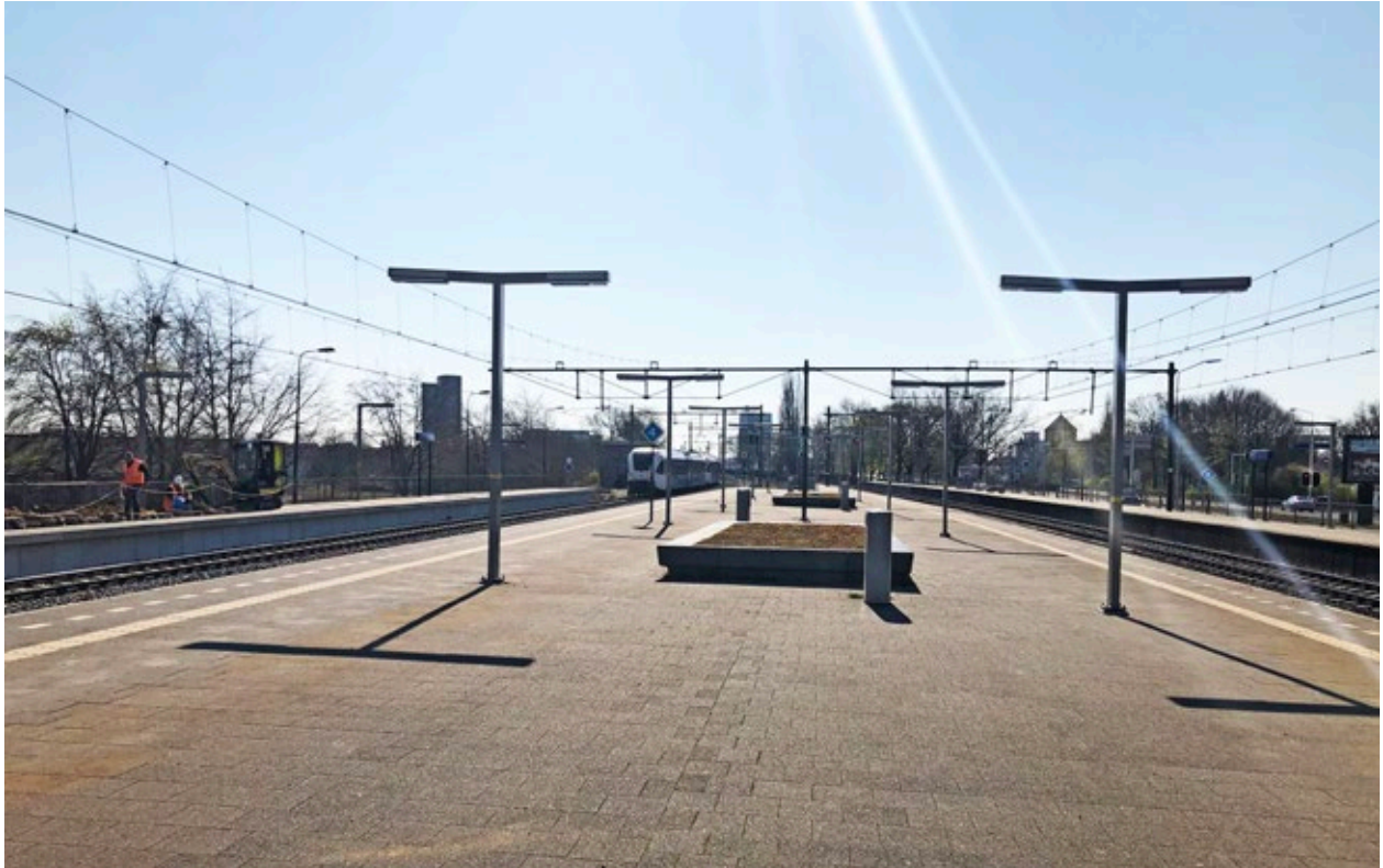
During the audit in April 2020. At the top, the dimming sensors were not yet installed.
